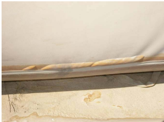
Figure 11: Example of major blistering. Multiple blisters of various sizes and filled with fuel.
