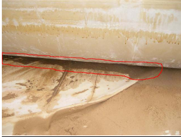
Figure 3: Example of a Class IV leak. The dirt within the red outline is saturated with fuel from three Class IV leaks underneath the tank. There were three patches put in place that stopped the leaks for eight months. When the tank started leaking again the leakage areas were cleaned and patched again but this time the patching failed and continued to leak. The tank was removed from service.
