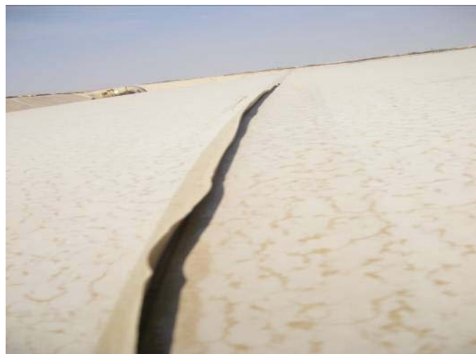
(Figure 10: (NOTE: APPARENT SEAM SEPARATION) - Some manufacturers will use a protective tape seal the seam edge. This is not considered a seam separation where the tape is no longer adhering to the tank. This condition warrants monitoring but shall not change the BRAG status until leakage is exhibited.)
