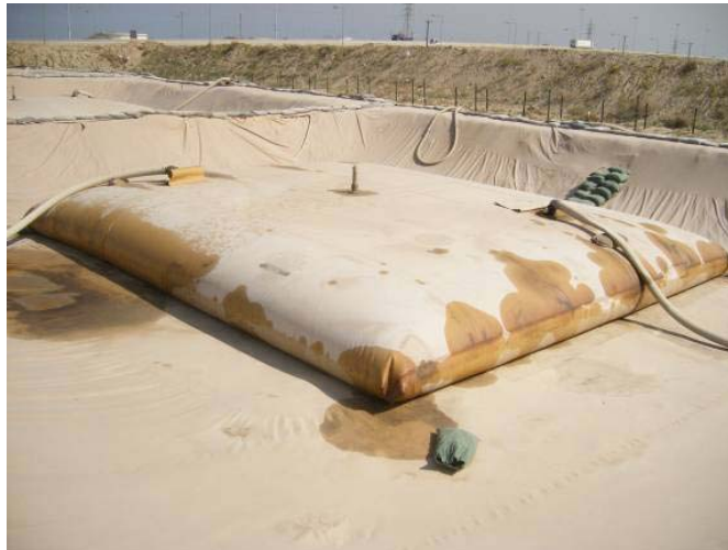
Figure 6: Example of non-repairable seam leakage. This tank was drained and taken out of service. BRAG status BLACK
