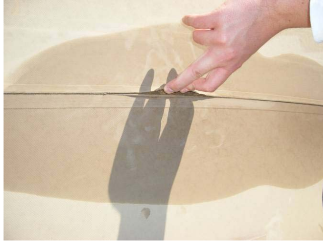
Figure 9: Example of a seam separation showing signs of Class I leakage.
