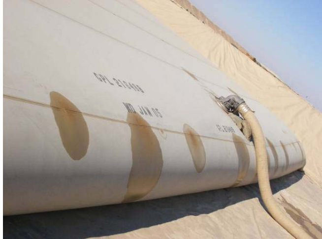
Figure 5: Example of multiple Class I/II leakage greater than 12” in diameter along the same seam line. BRAG status RED.
