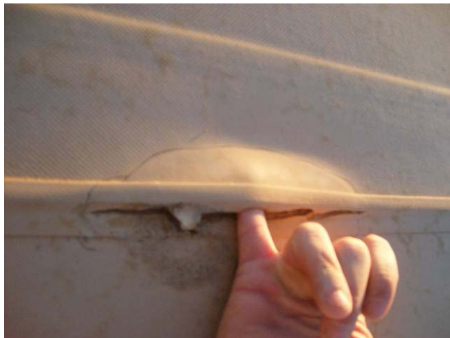
Figure 8: Example of a minor Seam Separation (less than a 1/3 width of the overlap of the fabric panels) with no signs of leakage.
