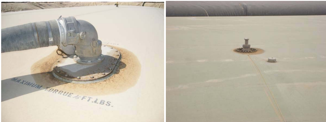
Figure 12: Example of Filler/Discharge Assembly (left) and Vent Fitting Assembly (right) showing signs of leakage. BRAG status Amber as shown, but track using fabric panel inspection criteria.
