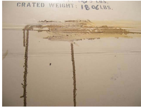
Figure 4: Example of a Class III leak. This leak was repairable making its BRAG status AMBER.
