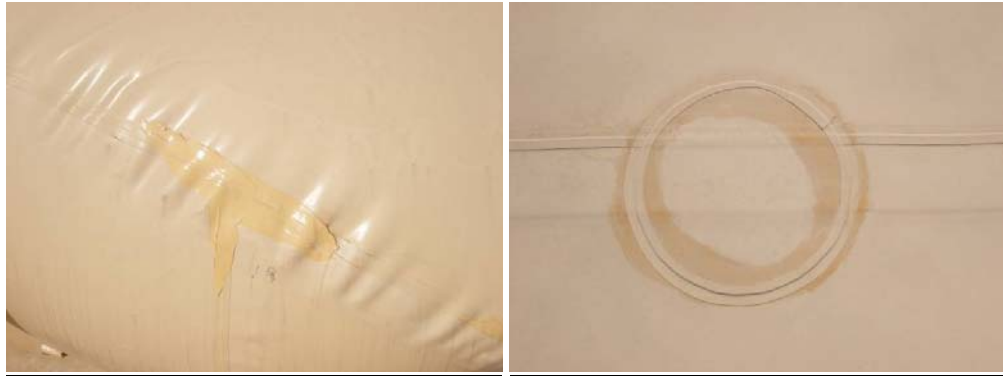
FIGURE 1. Two examples of manufacturer repairs/patches not considered deficiencies during the baseline inspection. These types of repairs/patches do not affect the BRAG status, but their location shall be noted on the BSTR for future monitoring and inspections.
