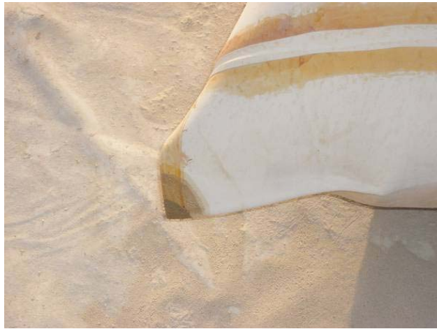
Figure 7: Example of a Class I leakage on a pointed corner tank. Some tanks have rounded corners. Placing a mechanical clamp may slow the leakage, but shall be cause to elevate the BRAG status and further monitoring.
